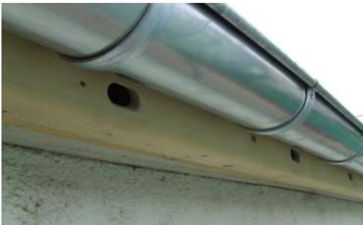
A simple timber box, with internal partitions, that has been fitted under and behind the gutter to form a continuous array of Swift nest places. The entrance holes are sized to resist access by Starlings.
